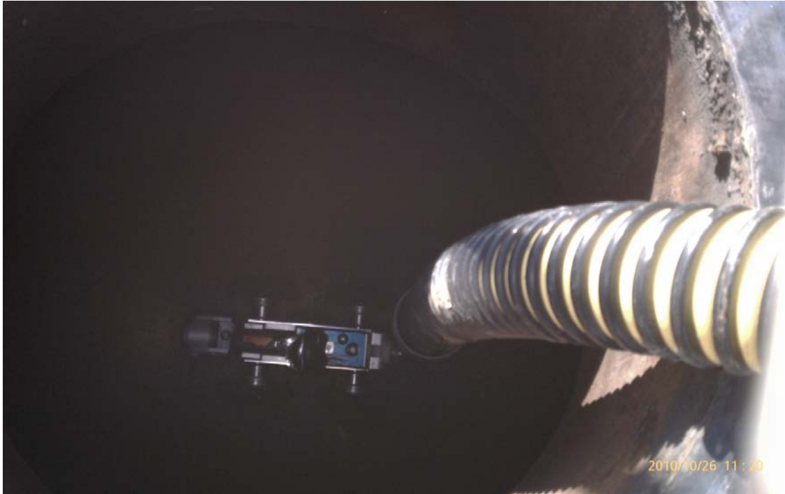
Figure 1. Video Inspection Rover In Pipe
